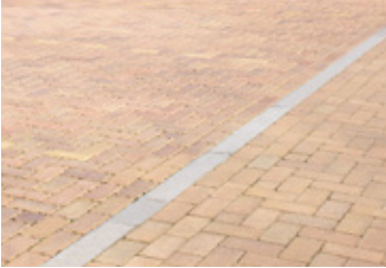
Pre-cast Concrete Edge
